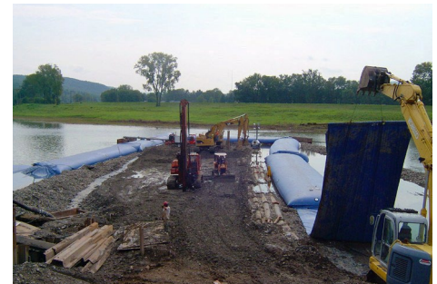
Chemung County Sewer Districts Chemung River Siphon Crossing City of Elmira, NY
