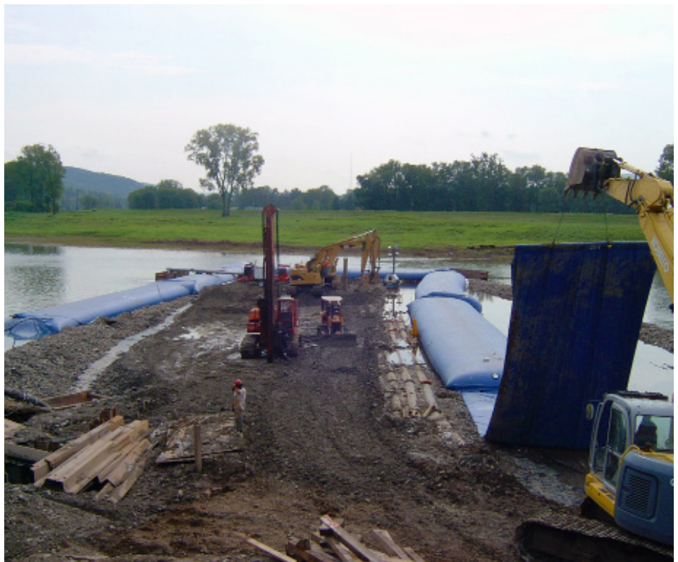
Chemung County Sewer Districts Chemung River Siphon Crossing, City of Elmira, NY
