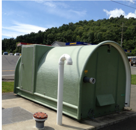
Chemung County Sewer Districts Wygant Sewer Pump Station Town of Horseheads, NY
