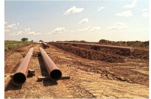
Natural Gas Transmission Pipeline Friendsville, PA
